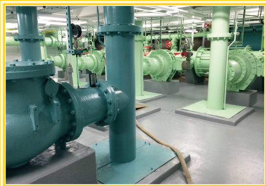
Water Treatment Plant Lower Water Room
